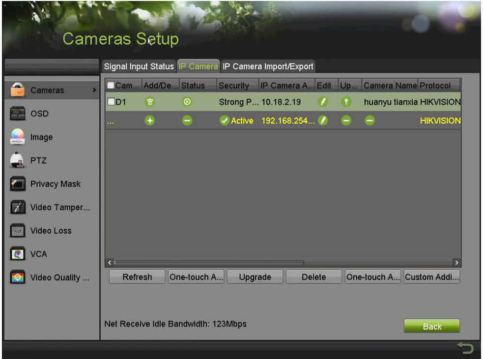
Figure 2, IP Camera Management Interface
